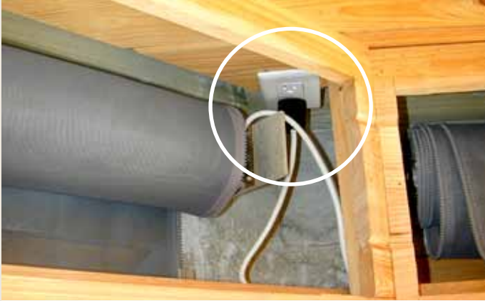
Duplex electrical outlet installed inside the cavity outside the working area of the screen's roller, mesh and motor
